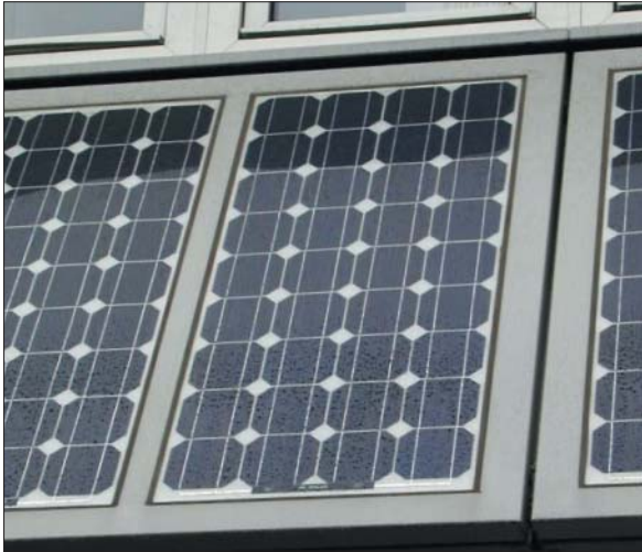
Photovoltaic cells are still developing but can make a useful contribution to the power needs of a building as here in the University of Northumbria
