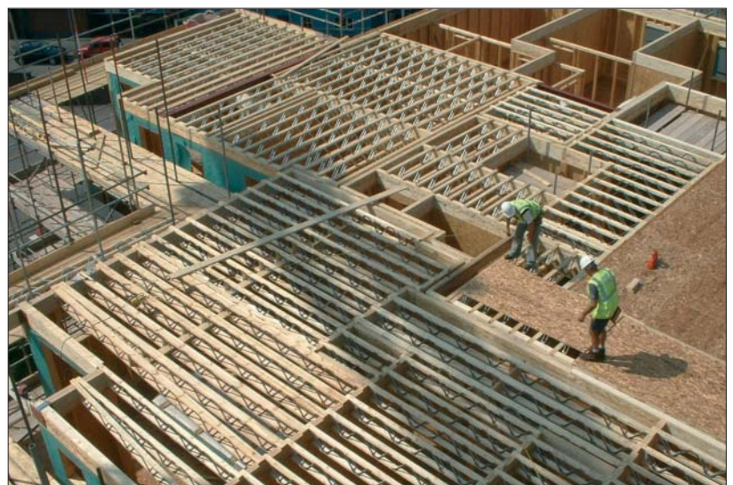
Fig 4. Seven-storey timber-framed structure designed by Chiltern Clarke Bond Ltd at Newcastle-under-Lyme for Taylor Lane Timber Frame Ltd s which used top-hung open web joists supported on a rim beam
