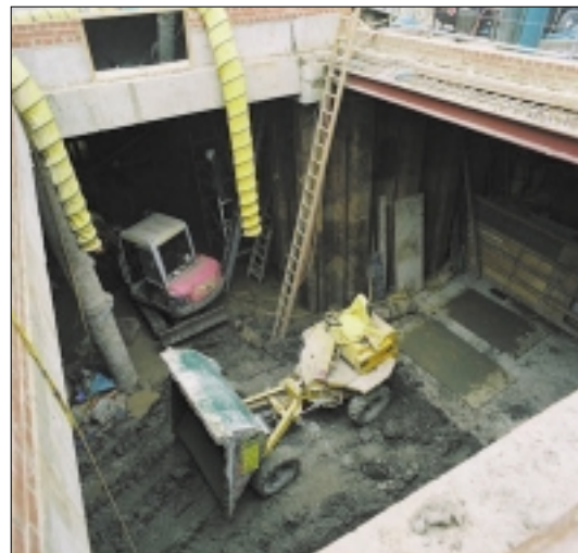
860m 2 of sheet piling was installed to form a basement with a plan area of 280m 2
