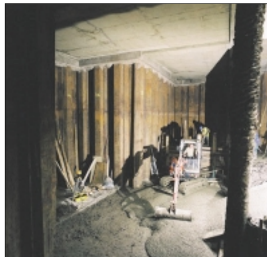
The sheet pile walls act as a retaining structure and carry axial loads from the superstructure
